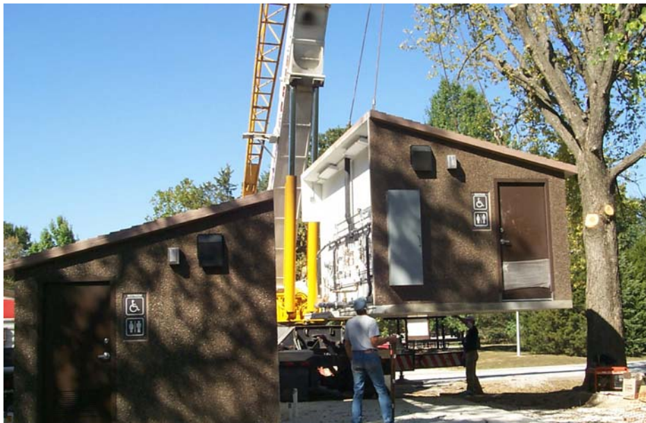
Photo K-4. Prefab unisex shower house. Nemo Park, Pomme de Terre Lake, MO. Installation of a prefab building shows some advantages of using commercially available units ( Paras. 1.21 and 3.5.2 )
