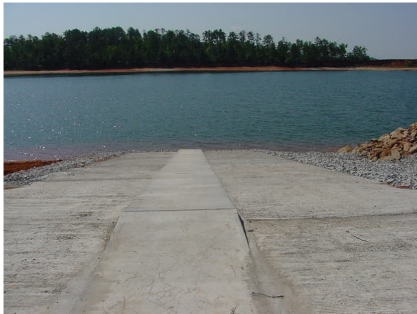
Photo N-2. Two-lane boat launching ramp. Scotts Ferry Boat Ramp, Thurmond Lake, SC. Courtesy dock is provided, but out of photo ( Table 5.8 )
