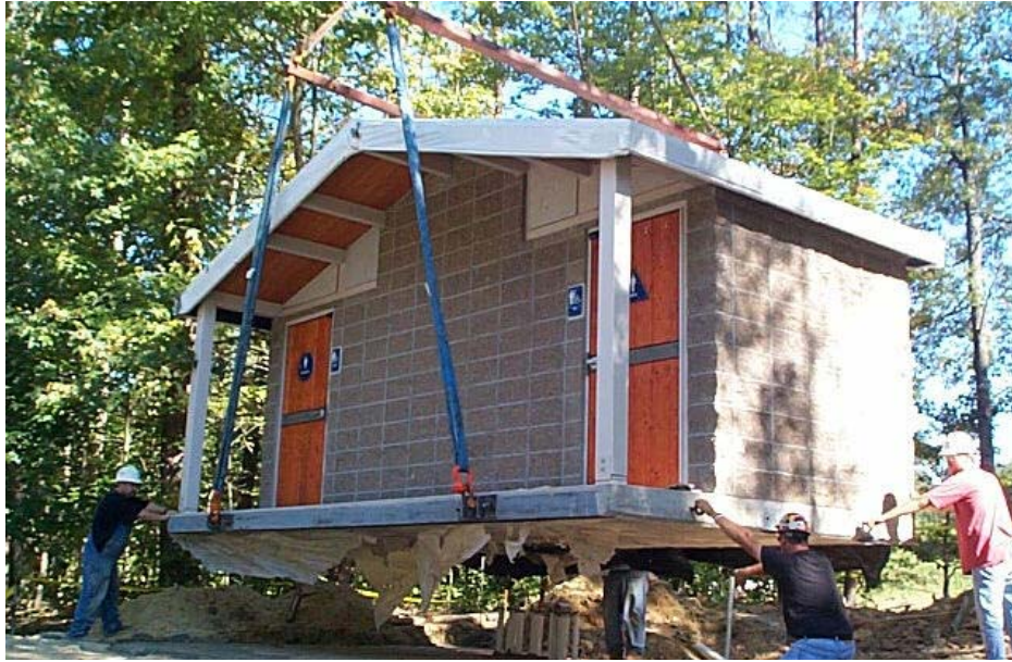
Photo K-3. Prefab restroom building. High Bank Recreation Area, Cave Run Lake, KY. Installation of a prefab building shows some advantages of using commercially available units ( Para. 1.21 )
