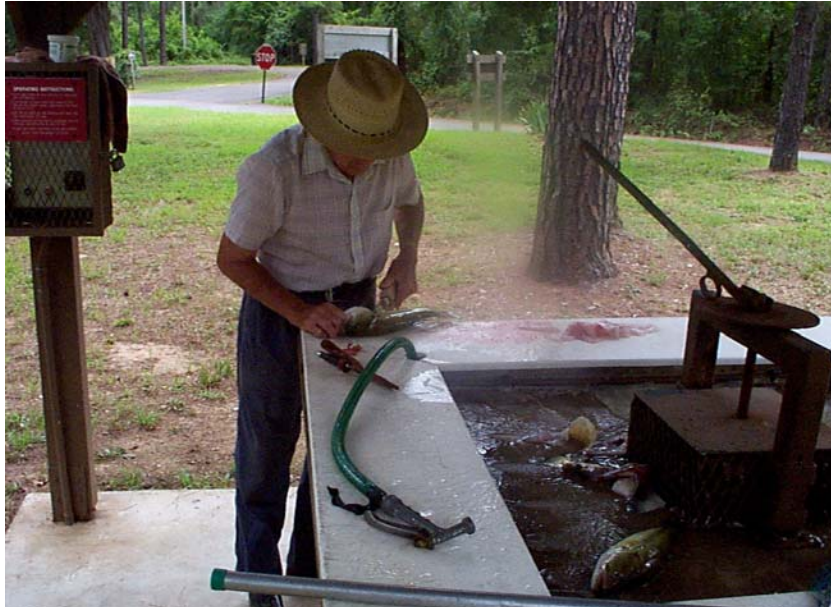
Photo L-3. Customer using fish-cleaning station. Carter Cove Park, Nimrod Lake, AR. This station includes two water hoses with spray nozzles, a 2-hp grinder with timed start/stop switch and custom cover (fish remains go into septic tank and leach field), GFCI receptacles, and night lighting ( Table 3.10 )
