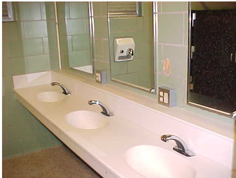
Photo K-6. Sinks incorporated into countertops. North Fork Campground, Rough River Lake, KY. Customers like the additional counter space. Also note that a GFCI protected outlet is provided for every two sinks, and motion-activated faucets have been included (Tables 3.4 and 3.5 )
