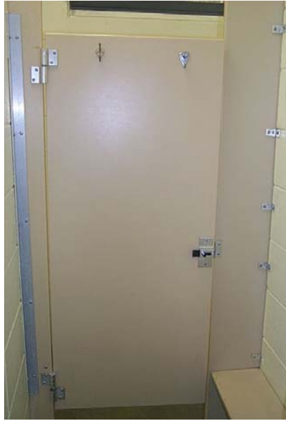
Photo K-9. Individual dressing area. Redman Creek Campground, Wappapello Lake, MO. Dressing area for shower stall has door with privacy latch, includes bench and clothing hooks. Shelf large enough for toiletries not visible in photo (Tables 3.4 and 3.5 )
